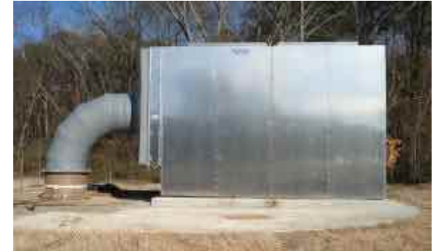
Parallel Bed Scrubber (<math><70.000\text{ m}^3/\text{h}</math>)
