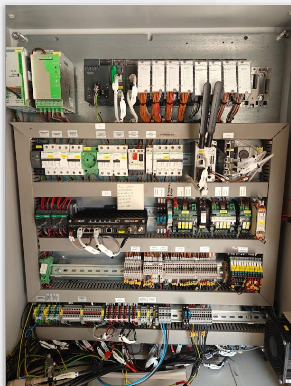
Armario telecontrol renovado
